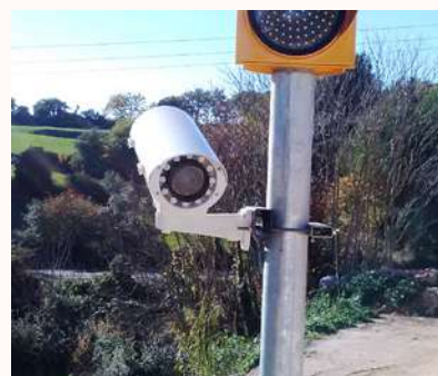
CCTV AND ANPR CAMERAS
